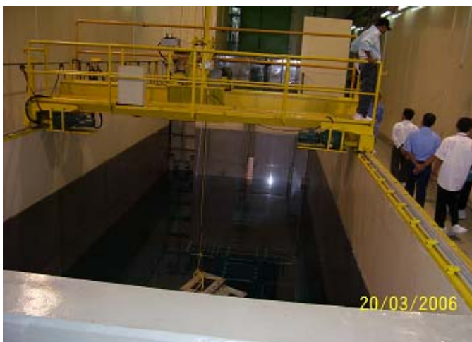
Fig. 4. Spent Fuel Storage Facilities
